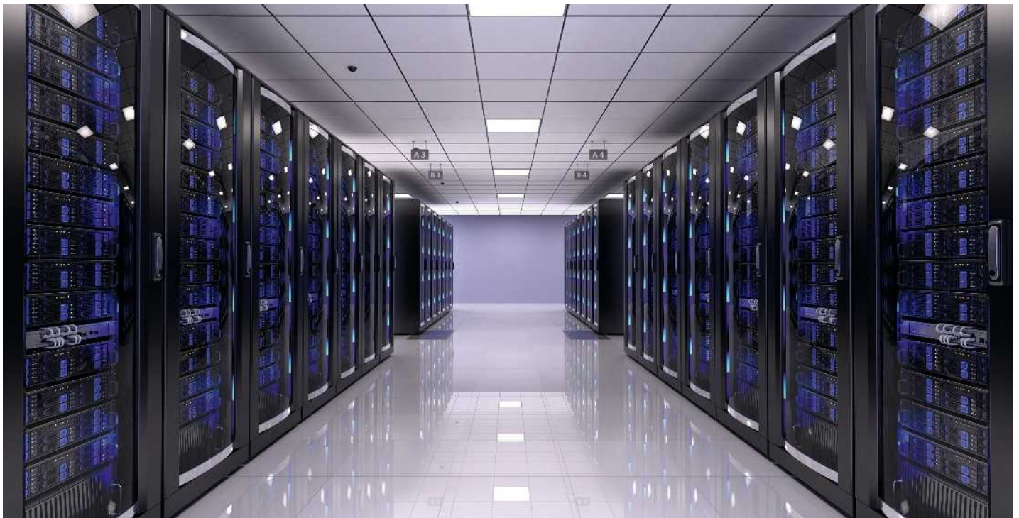
Fig. 68: Data center with a DC power supply system with linear source characteristics
